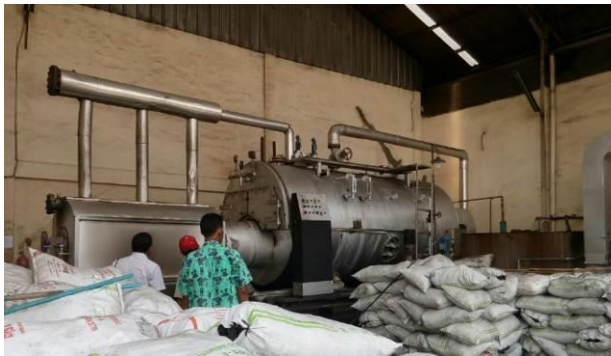
Follow up visit to noodle factory at boiler section
