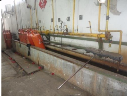
Heating LPG tubes with condensate
